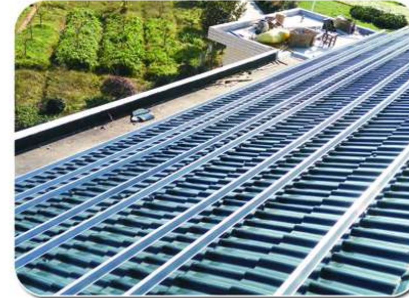
500KW SFS-PR-01 Tile Roof Mount(Australia)
