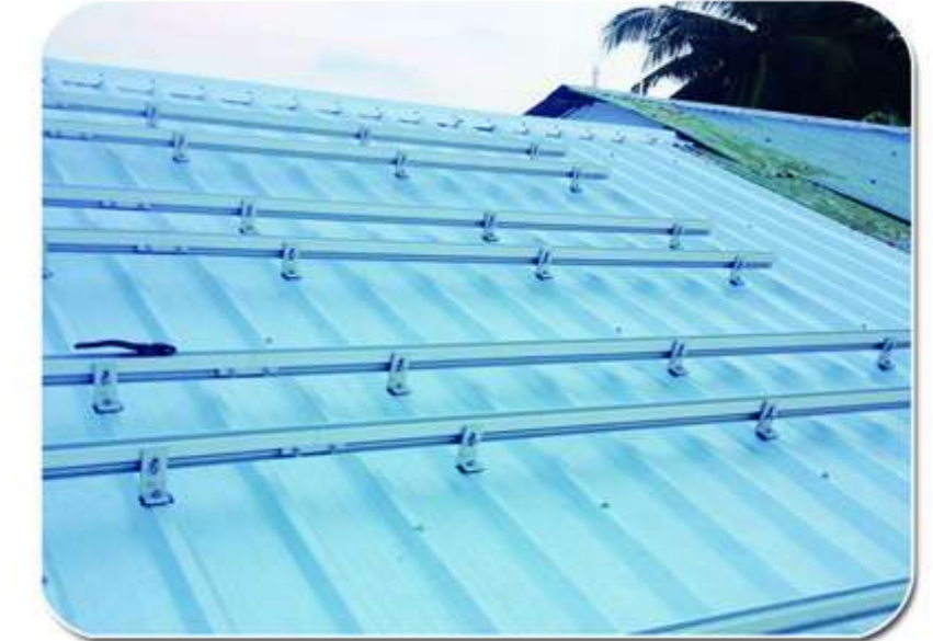
300KW SFS-PR-01 Tin Roof Mount(Philippine)
